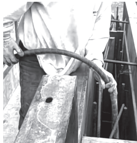
Figure 5.13: A vibrator is inserted into concrete from the top of the formwork
