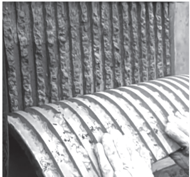
Figure 5.10: Form liner is peeled away to reveal ribbed concrete surface, Milstein Hall, Cornell University, designed by Rem Koolhaas-OMA (from the Construction of Milstein Hall Part 2 Substructure video by the author at https://jjonochshorn.com/scholarship/videos/milstein/ )
