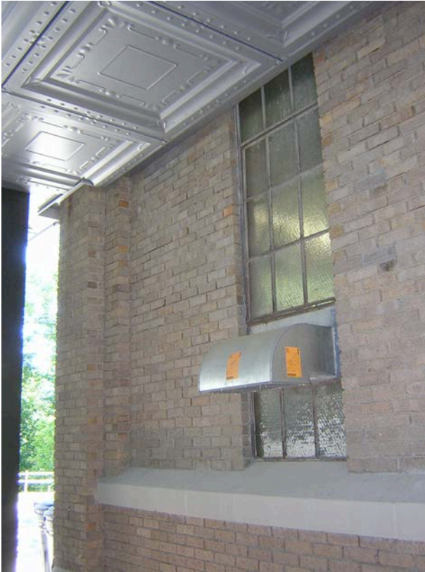
Figure 3. Lack of opening protectives in fire barrier between Rand and Milstein Hall (photo by J. Ochshorn, June 2013)
