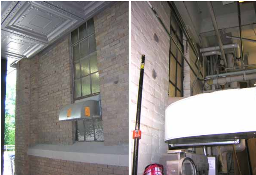
Photos taken today showing Rand Hall exhaust duct and window from the outside, directly under Milstein Hall (left); and from the inside of the Rand Hall Wood Shop (right).
